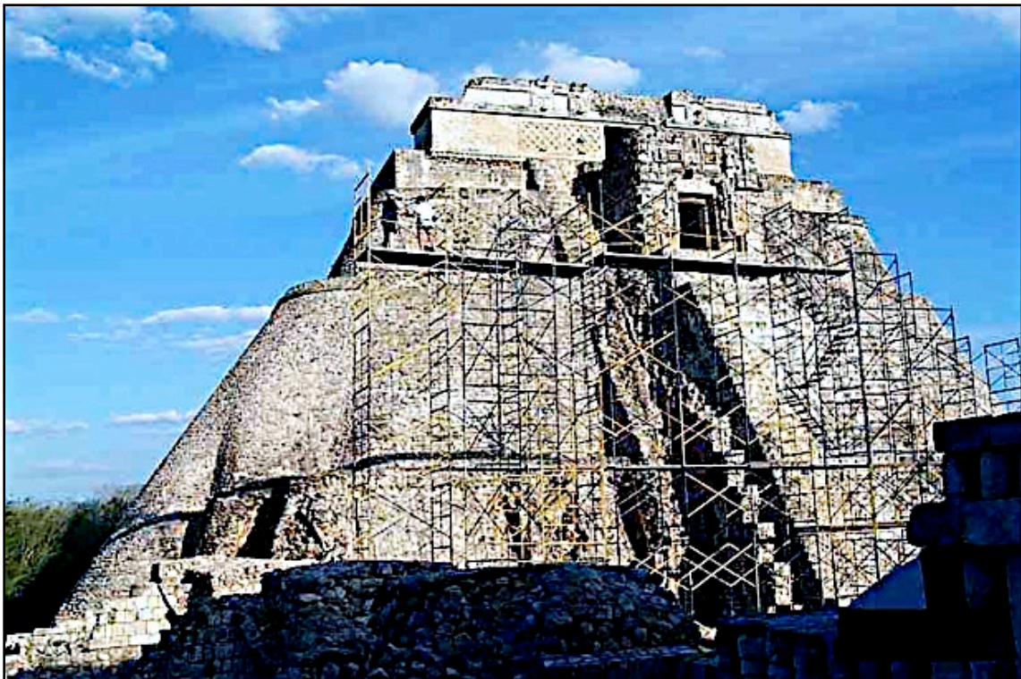
Figure 13. Scaffolding for photographing the upper part of the west façade of the Adivino Pyramid. 1999. Bryan and Clowes are photographing at the 14 meter level. Photograph by Roberto Centeno.1999.
