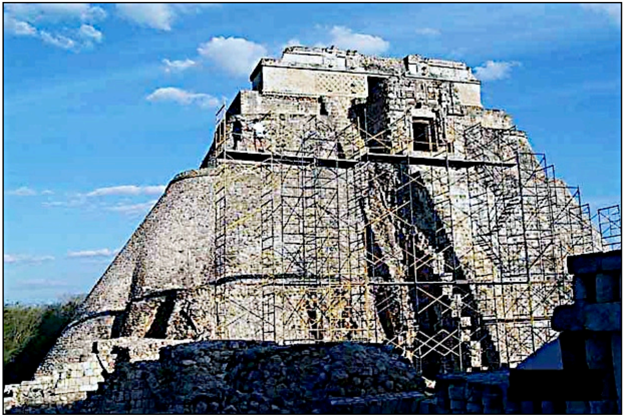
Figure 25. Scaffolding for photographing the upper part of the west side of the pyramid. Paul Bryan and Michael Clowes are photographing in the upper left corner of the scaffold. Pic: Roberto Centeno L., 1999.
