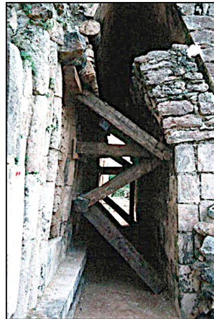
Figure 19. Emergency wood shoring within the tunnel under the west stairway. Shoring was later replaced by stone and concrete for greater stability. Note stairway separation from main structure in upper right corner. Pic: L. G. Desmond, 1989.
