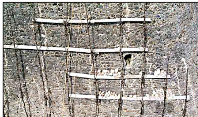
Figure 23. Scaffolding for inspection of cracks in stonework, and the interior of pyramid on south side. Pic: Roberto Centeno, 1999.
