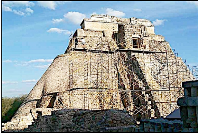
West facade of Adivino Pyramid at Uxmal. Scaffolding with Paul Bryan and Mick Clowes making 3-D stereo photographs for close-range photogrammetry documentation. Pic: Roberto Centeno Lara. 1999.
