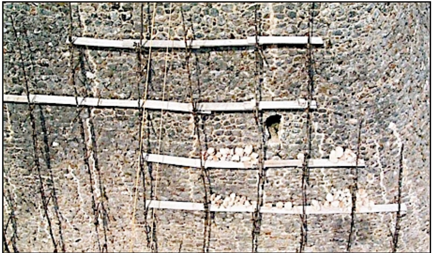
Adivino Pyramid south facade. Cracks are filled with light colored concrete. Exploration hole was dug by archaeologists to research structural instability, and develop a strategy to prevent further damage. Pic:Roberto Centeno Lara. 1999.
