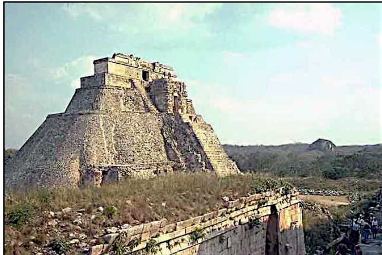
The Adivino Pyramid at Uxmal from the northwest. Note filled vertical cracks in the facade. Pic: L. G. Desmond. 1999.
