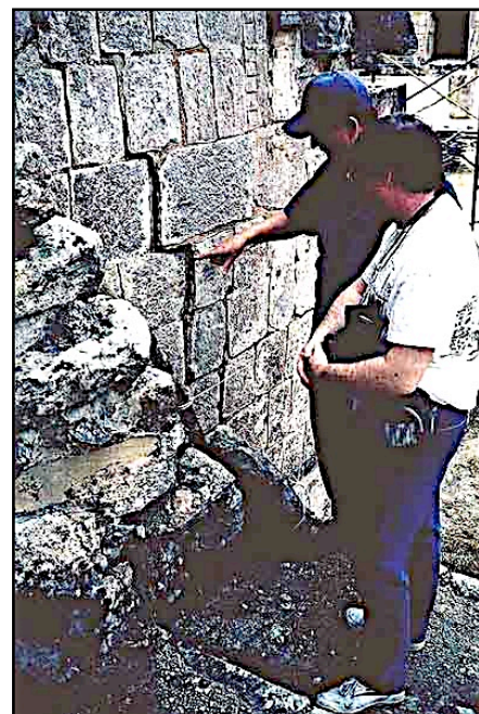
Inspecting cracks in the west stairway of the Adivino Pyramid, Uxmal. 1999
