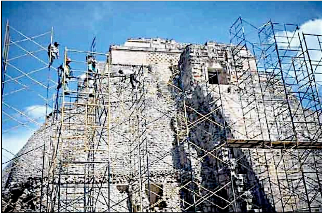
Scaffolding being erected for photographing the west facade of the Adivino Pyramid. Pic: L. G. Desmond. 1999.
