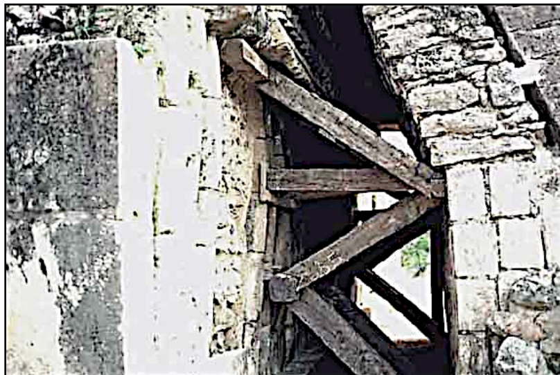
Shoring under west stairway to prevent collapse. Note plaster patch upper right corner used to detect separation of stone. Pic: L. G. Desmond. 1989.
