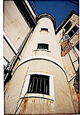
Photo 7. Tower of Fenice Theater and apartment building. Cracks are noted in the window area.
