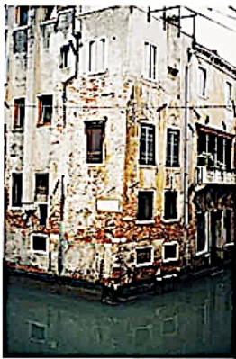
Photo 11. Building at the intersection of Rio delle Veste and Rio delle Outroche showing deterioration of building fabric. This is an area of high boat traffic.
