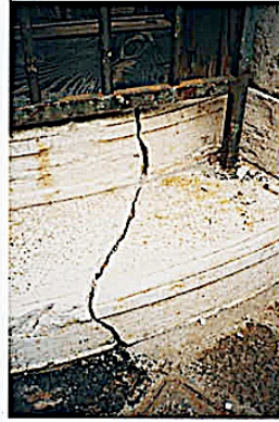
Photo 6. Entrance to Fenice Theater showing damage to stone work.
