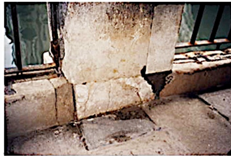
Photo 9. Damage to base of column of apartment building.
