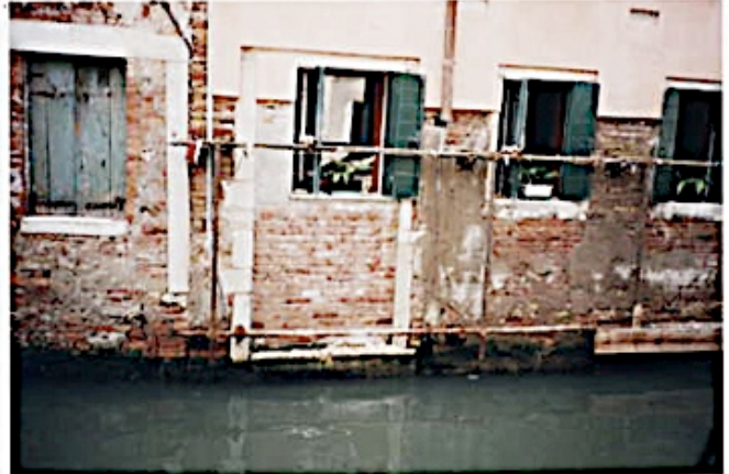
Photo 27. Fabric of residence on the south side of rio di Sant' Andrea undergoing repair.
