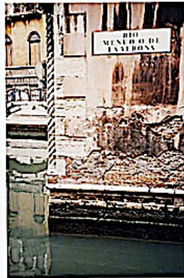
Photo 12. Corner of rio Manuo and della Verona (east side) showing cracks and other damage to fabric of building.
