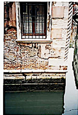
Photo 13. Corner of rio Manuo and della Verona (south side) showing cracks and other damage to fabric of building.
