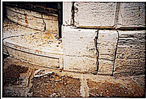
Photo 5. Base of Fenice Theater tower, entrance, and showing damage to stone work.
