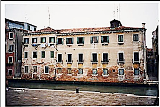
Photo 24. Canale dell' Arsenale, viewed to the west, showing damage to brick work on lower part of buildings about 100 meters from the Becino di S. Marco.
